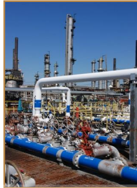
Lima Refinery (160,000 bbls/d)
